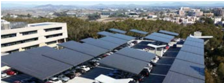
Photovoltaic panels on top of Hopkins Parking Structure provide energy and shade.
