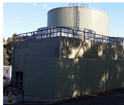
West Campus Cooling Tower.
