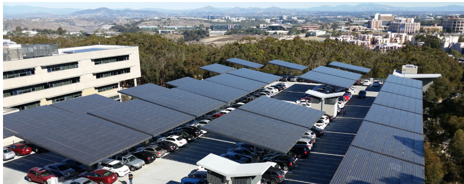
Photovoltaic panels on top of Hopkins Parking Structure provide energy and shade.
