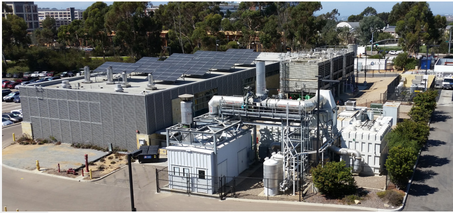
East Campus Energy Park.
