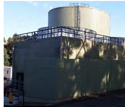
West Campus Cooling Tower.
