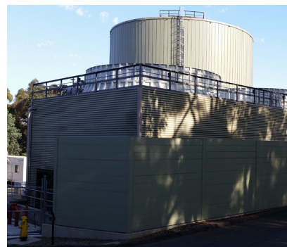
West Campus Cooling Tower.
