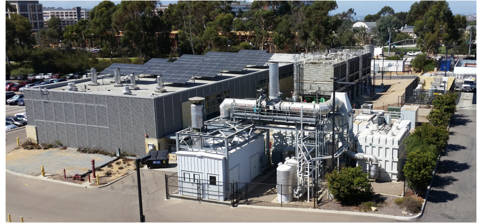
East Campus Energy Park.
