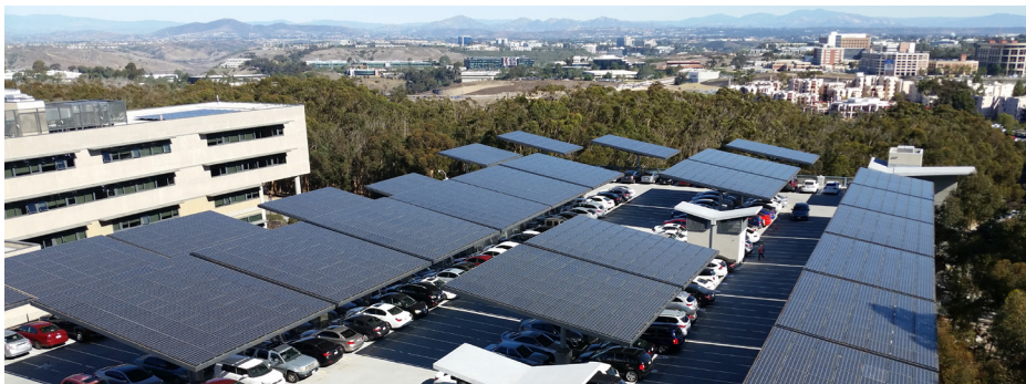
Photovoltaic panels on top of Hopkins Parking Structure provide energy and shade.
