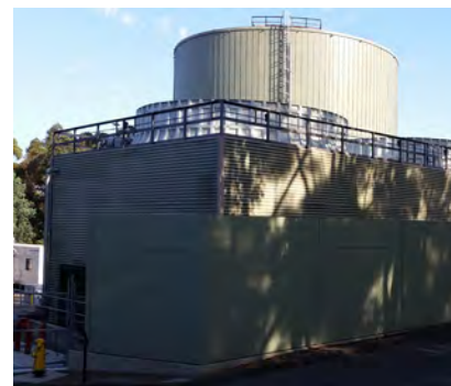
West Campus Cooling Tower.
