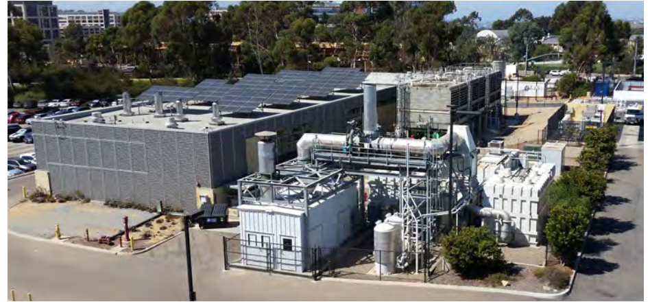
East Campus Energy Park.
