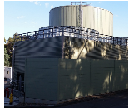
West Campus Cooling Tower.
