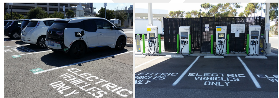
Electric vehicle parking and charging station on campus.
