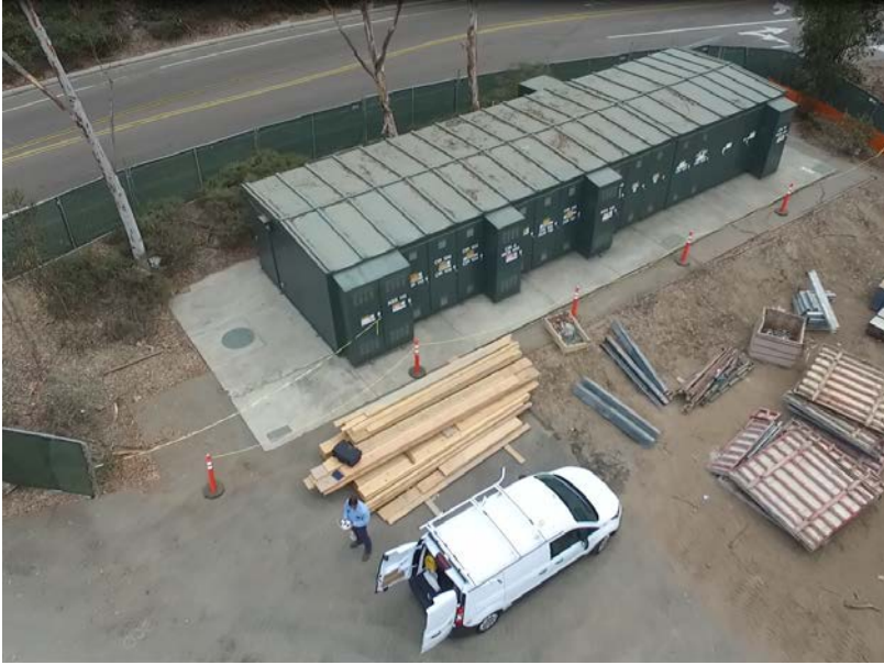
Existing Revelle Substation
