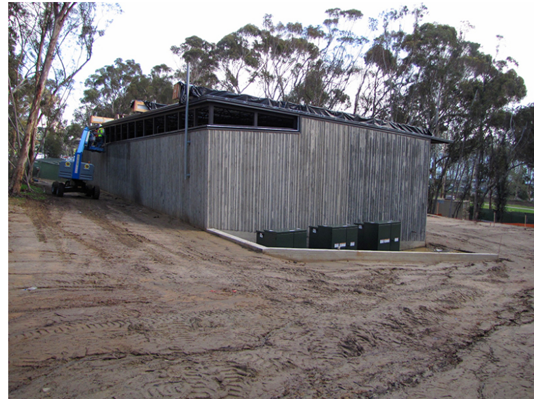
New Revelle Substation Building
