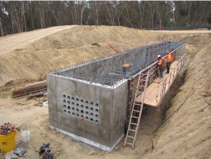
New Revelle Substation Vault
