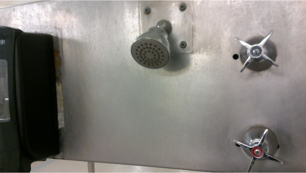
Shower head, knobs and stainless backing with heavy corrosion and dull finish
