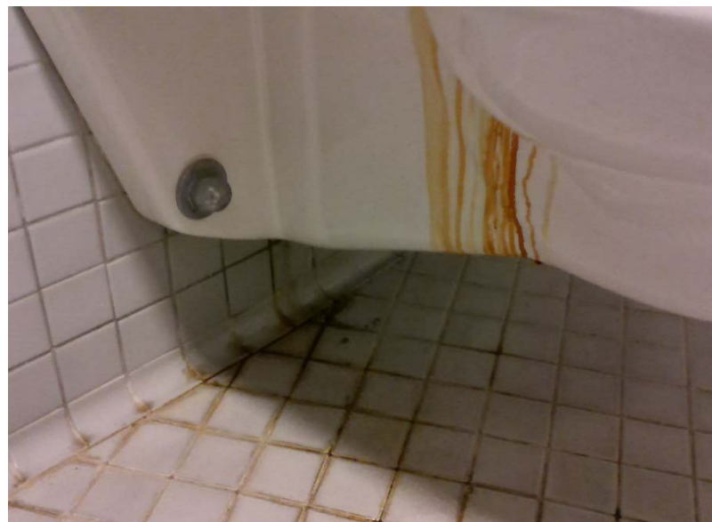
Toilet in need of scrubbing
