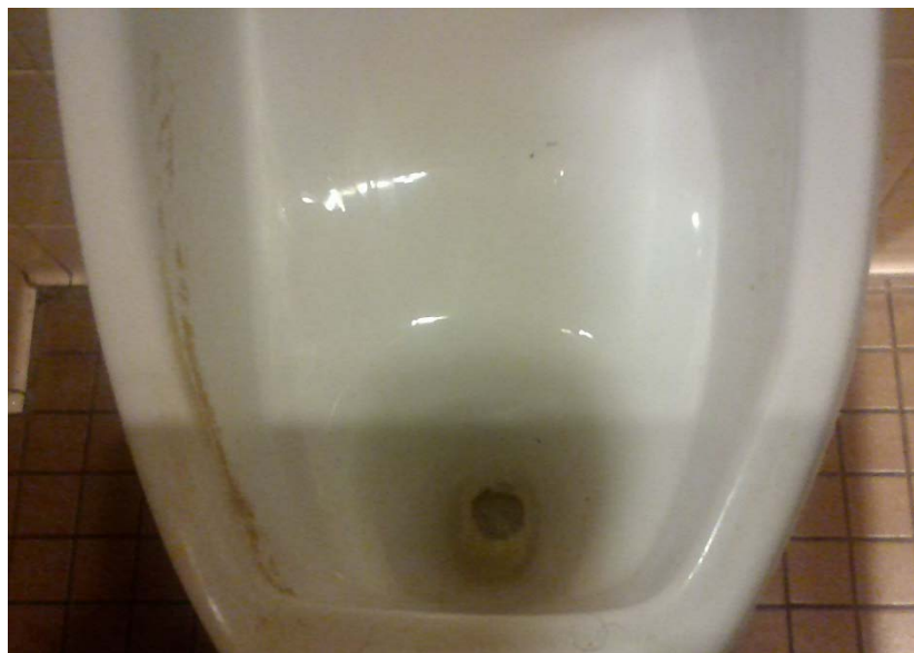
Urinal needing scrubbing
