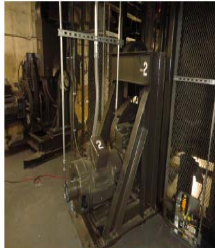
Elevator 2 machine - painted
