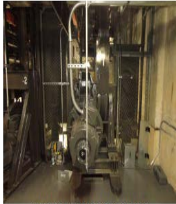
Elevator 1 machine with new motor
