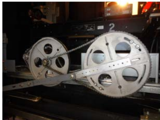
New GAL MOV FR closed loop door operators on all cars
